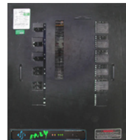
Strand Environ® rack with ENVY digital DMX control
