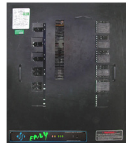
Strand Environ® rack with ENVY digital DMX control
